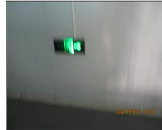
Photo of fire safety equipment Evacation signs.JPG
