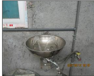
Photo of chemical storage room (if applicable) Eye washing.JPG
