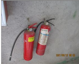
Photo of fire safety equipment Fire extinguishers.JPG
