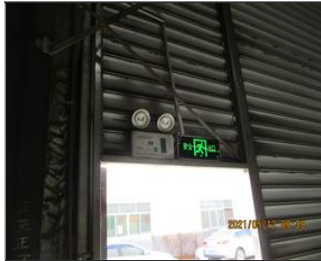
Photo of fire safety equipment Emergency lighting and exit.JPG
