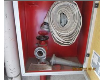
Photo of fire safety equipment Fire hydrant.JPG
